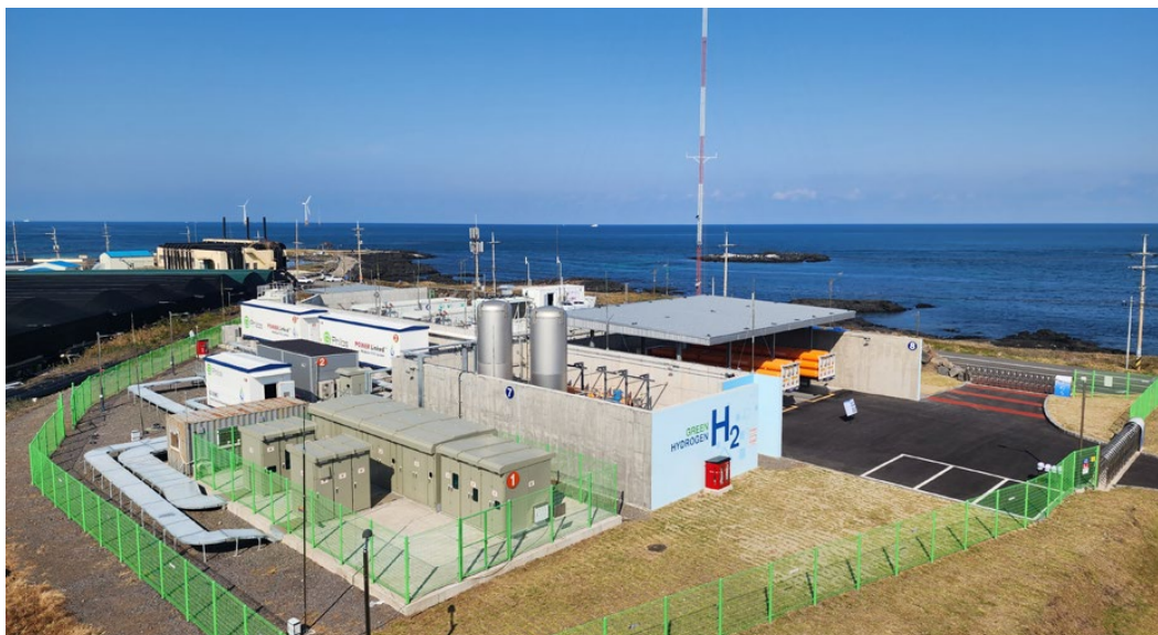
Figure 7. 3.3 MW Green Hydrogen Production and Storage System Site
