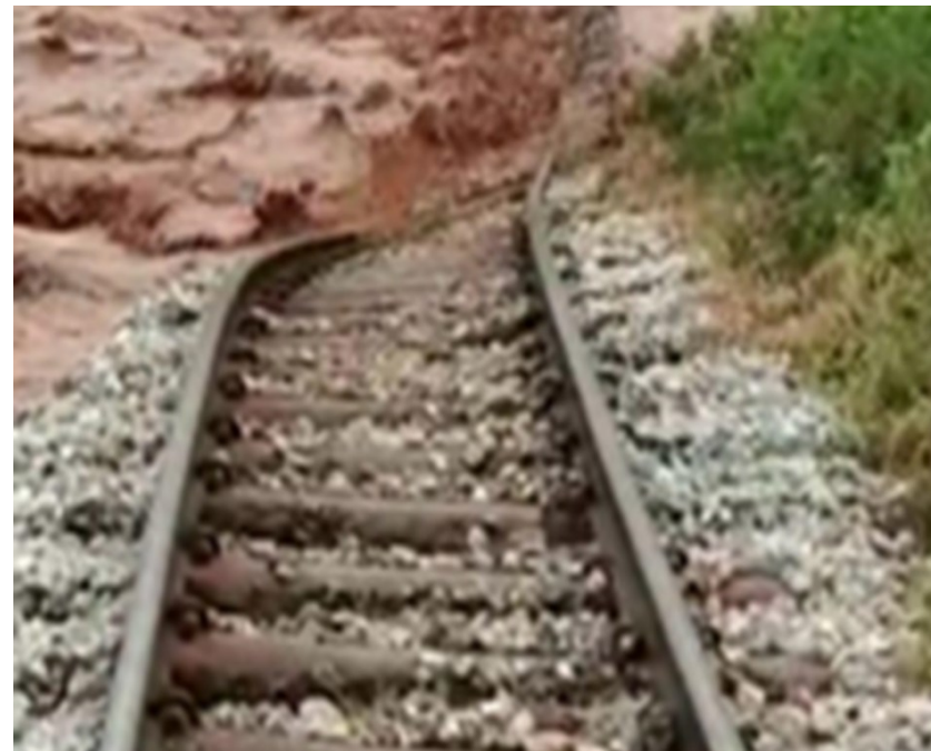
A flood- destroyed MGR railway track
