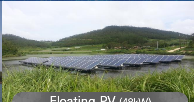
Floating PV (48kW)
