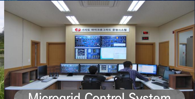
Microgrid Control System
