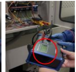
② Check abnormal status
