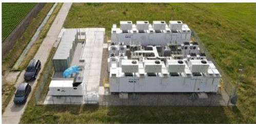
To bridge the gap between solar generation (middyay) and night-time charging large-scale BESS are needed to shift this generation.
